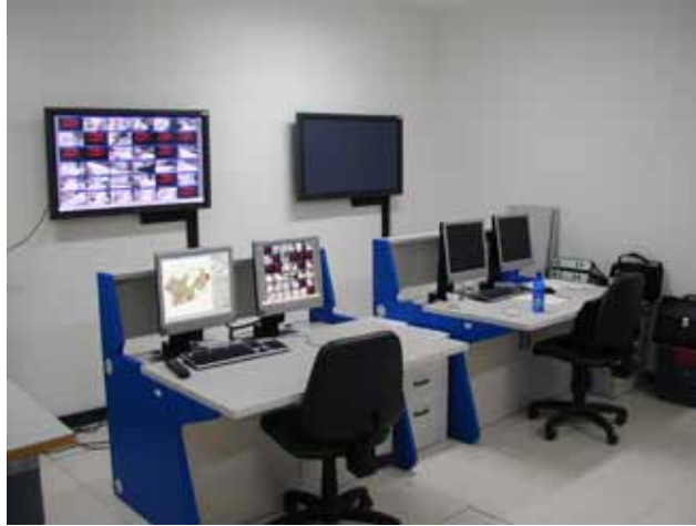
Figure 4: The main control room shall be neat, comfortable and with good perimeter protection and an effective access control (the Pompeii excavations main control room has a biometric access control device)
