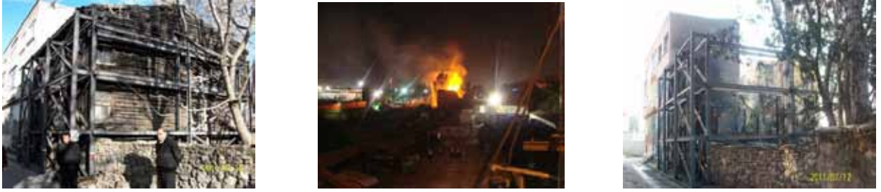
Figure 3: Focusing on a single point in planning risk management causes some second but important risks' being ignored. Despite the reinforcement was successful in preventing historical artifact's destruction included in the figure above, the building was exactly destroyed because of the fire (Resource: Gama Nurol Archive,2011)
